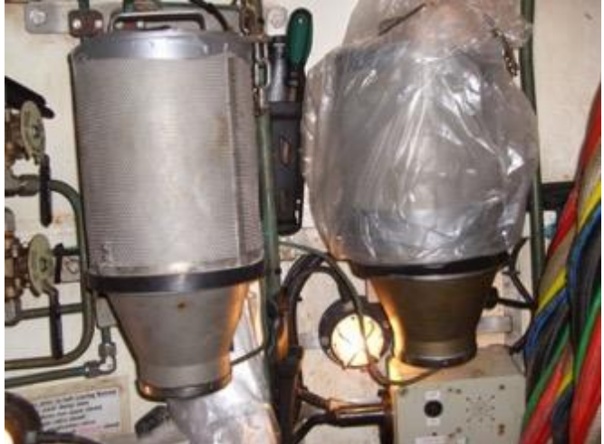
Bell CO 2 scrubbers
