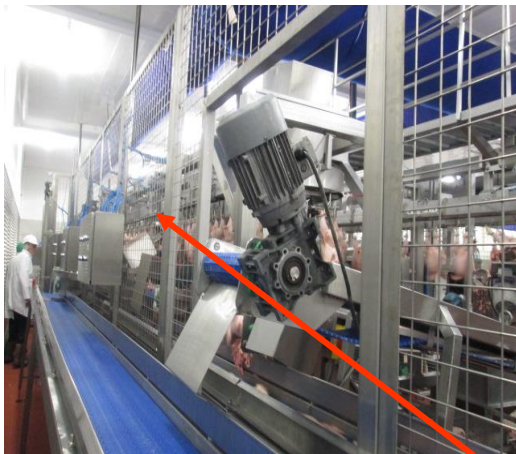
Fence Guard to Rear of Machine 12 metres in length!
