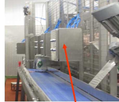
Air Motor Control Panel Line 2
